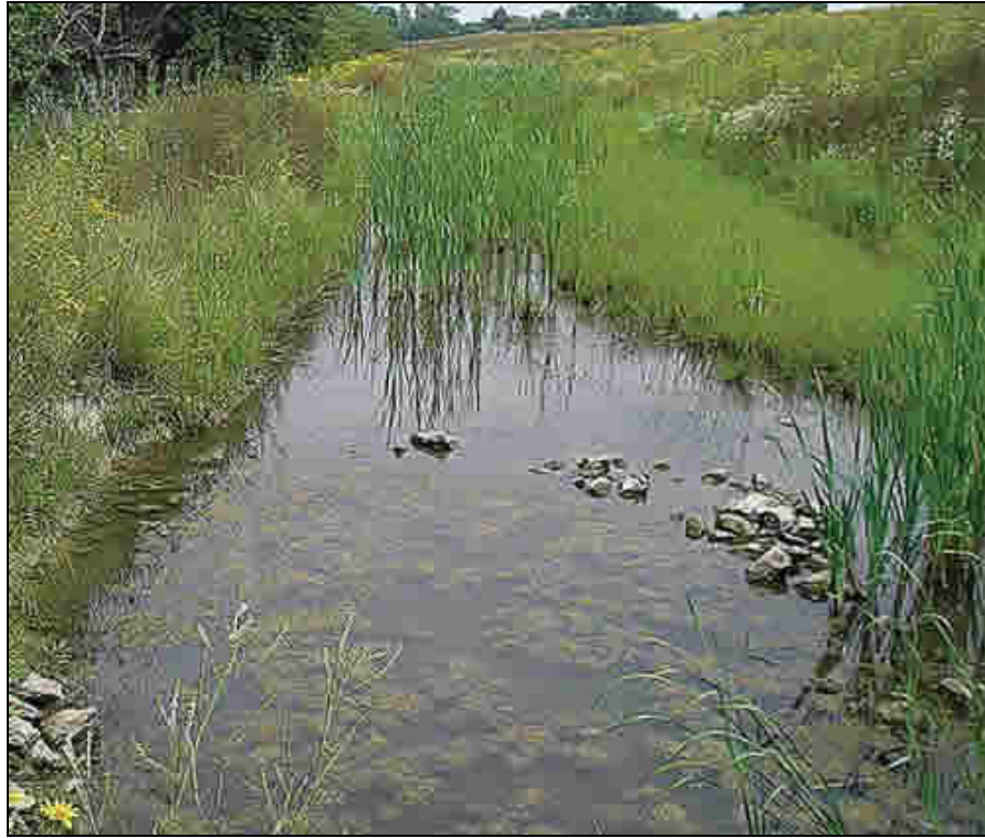
Photograph 4-4. Sediment Retention Structure
