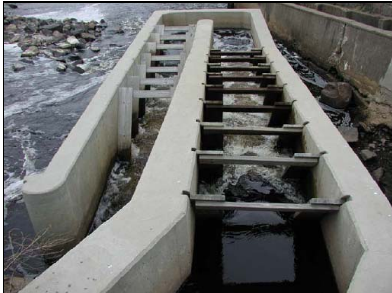
Photograph 3-6. Denil Structure at Ipswich Mills Dam, Ipswich, Massachusetts http://www.mass.gov/dfwele/dmf/publications/tr17_anad_p3_appendix.pdf
